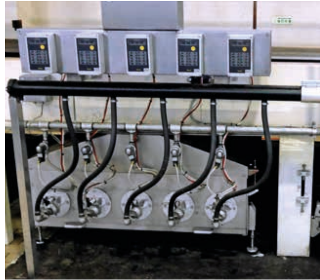
This is a dirt burning station at oven's exit, which did not work successfully and was consequently switched off.
