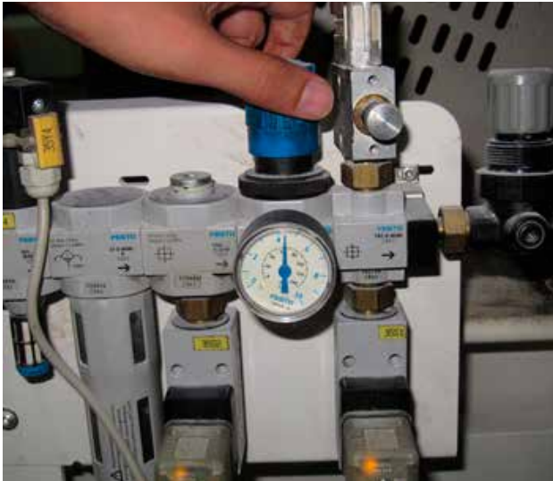
A too high tensioning of >4 bar
